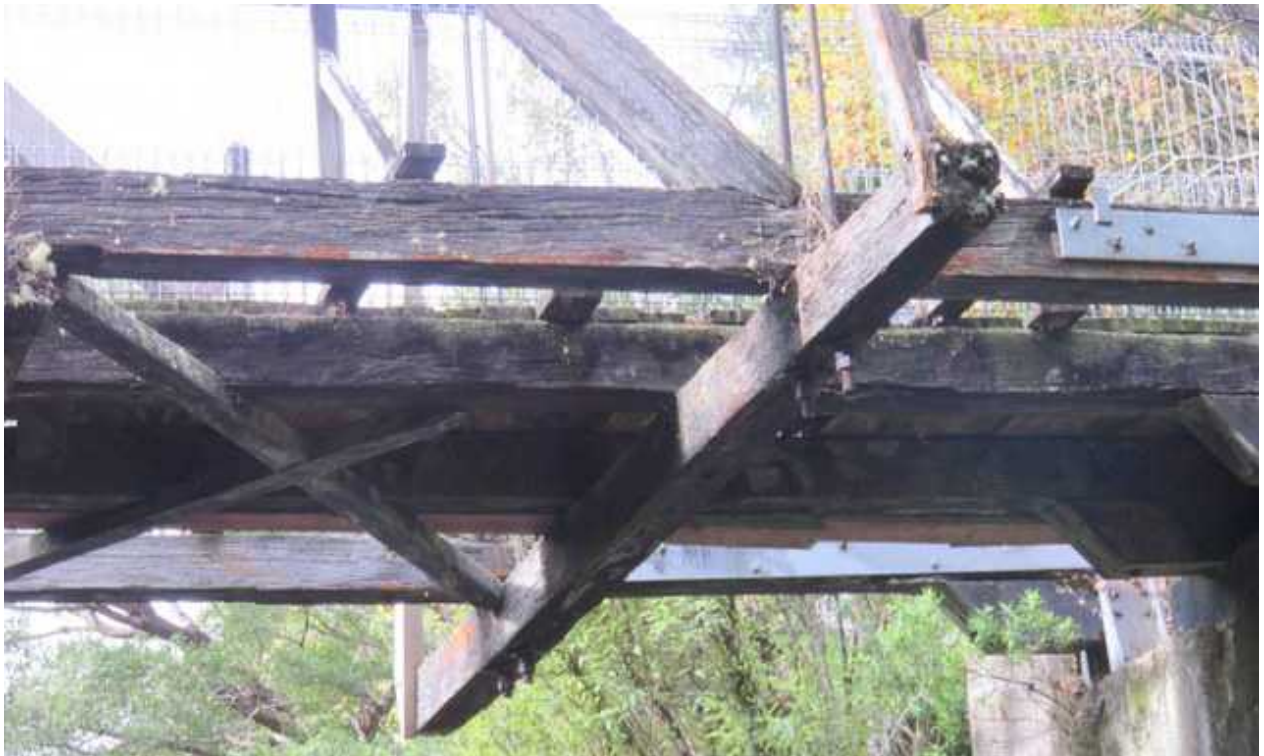
Illustration 21: Underlying deck structure (22 nd May 2020).
