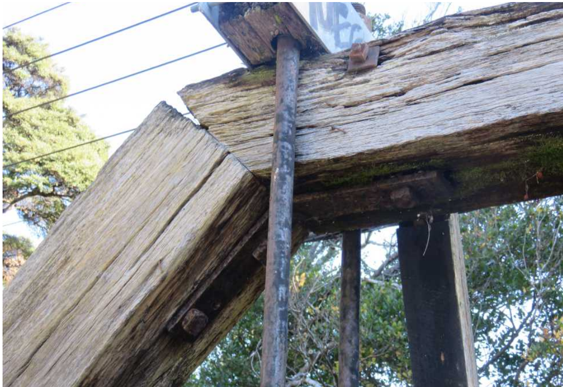
Illustration 24: Iron reinforcing plate underneath top chord and end post joint (9 th June 2020).
