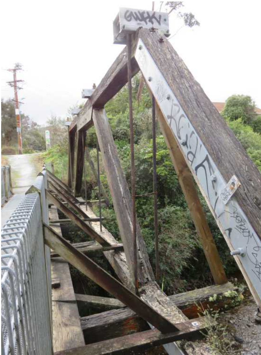
Illustration 32: Beechwood Lane bridge showing modifications to original timbers with resin filler in bottom chord, eastern side and galvanised, bolted reinforcing plates on south-eastern end post (22 nd August 2019).
