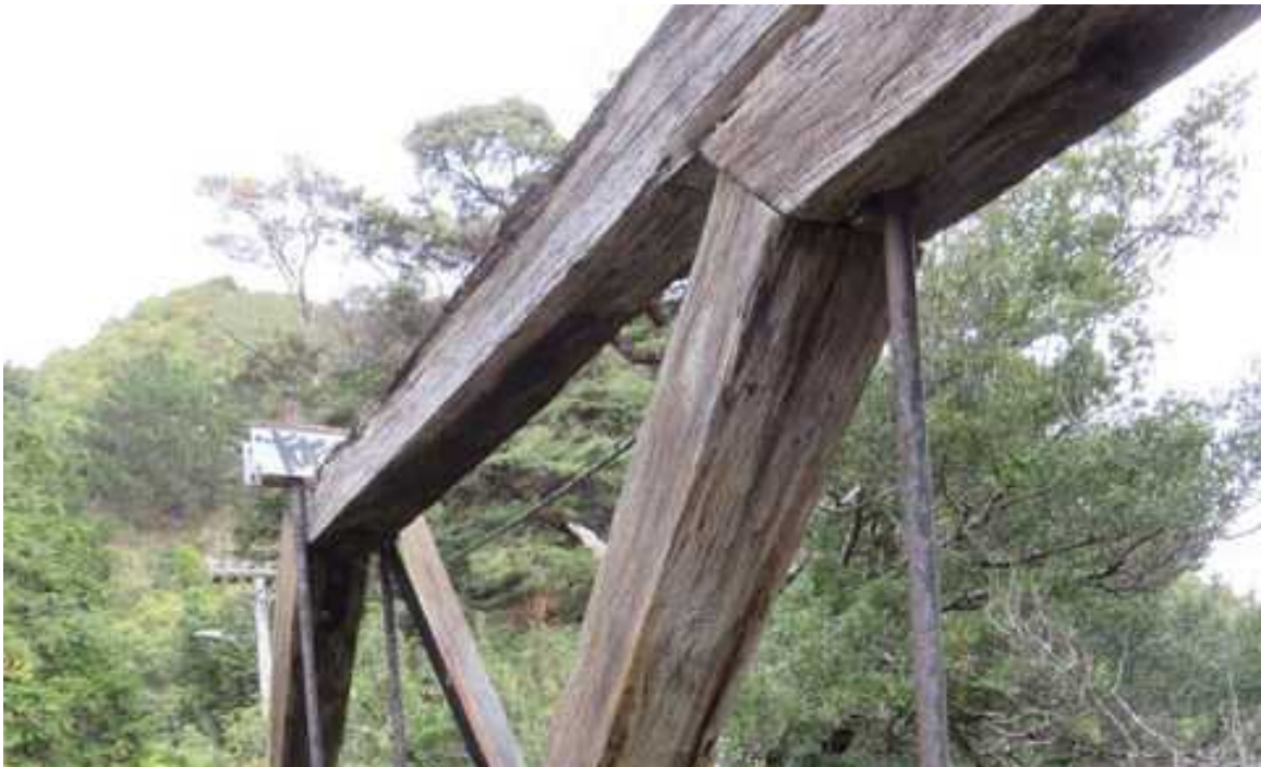
Illustration 23: Butt joint between transom and diagonal strut (22 nd May 2020).
