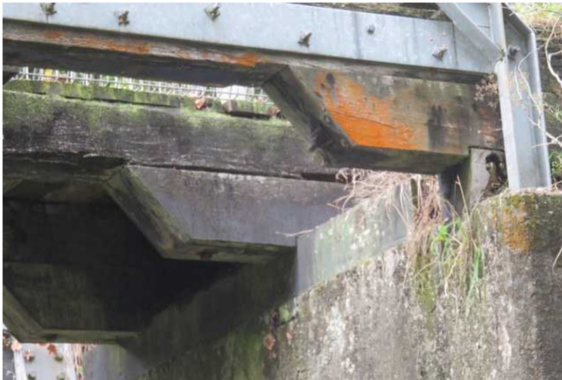
Illustration 30: Beams and stringers secured to concrete abutment at south end (22 nd May 2020).
